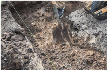
Map the preferred build area with a string line. Dig down to start building the foundation.
