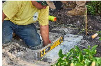
Lay the first course, making sure it's buried to provide a footer for your wall. Ensure level with torpedo level.
