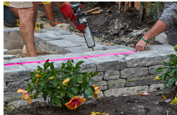
There should be two lines of Ladera, per course. Make sure the flat edges meet in the middle at the seam.
